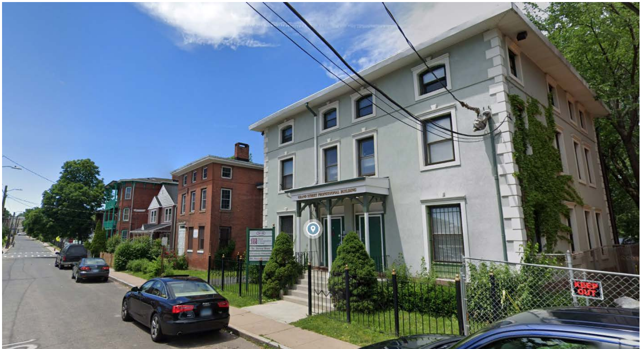
36-38 Grand Street, window hoods, casings, and sills restored, Google street view June 2019
