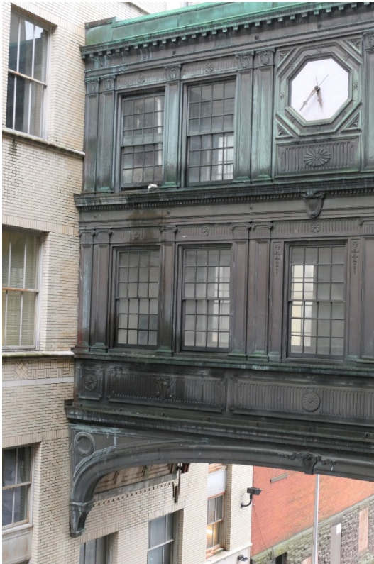
Figure 3. General atmospheric soil deposition and water staining on copper surfaces.
