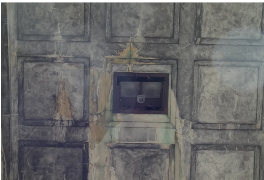
Figure 18. A flat panel in one soffit was removed to accommodate the installation of electrical equipment.
