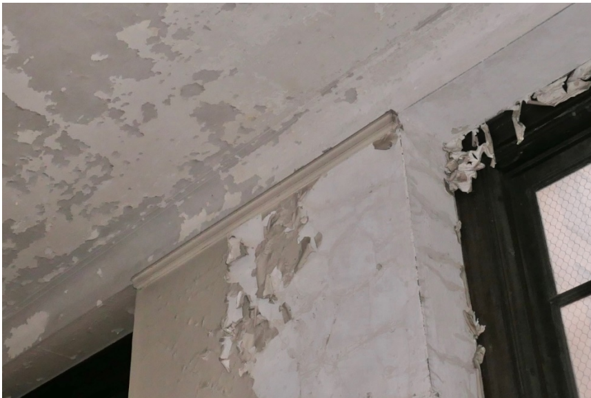
Figure 20. General atmospheric soil deposition and finish failure at the painted wood picture molding at the first level.
