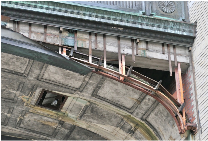
Figure 11. Missing copper cladding section and exposed underlying metal framing and concrete encasing of the steel structure on the west elevation.
