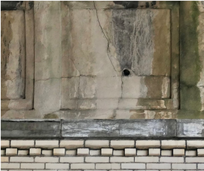
Figure 17. Surfaces losses and cracks at isolated locations in the cement plaster soffit.
