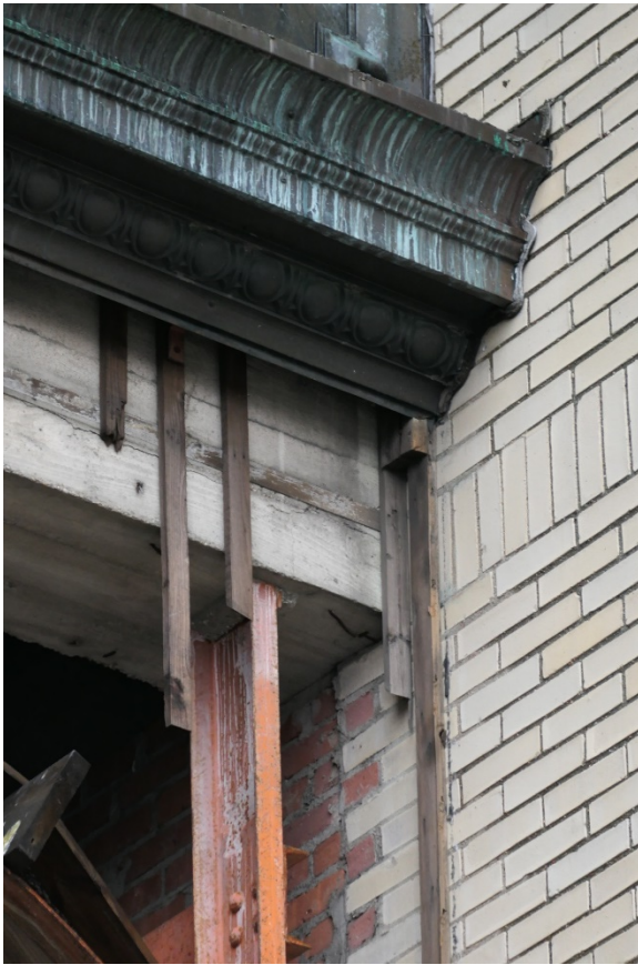
Figure 19. Water-damaged and displaced wood elements at the cladding armature.
