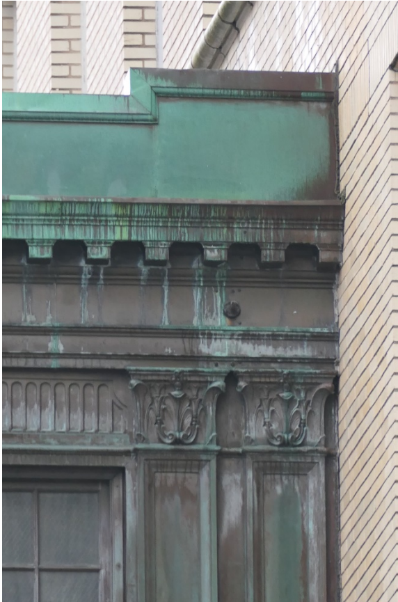
Figure 5. Water staining on copper surfaces at upper-level cornice.
