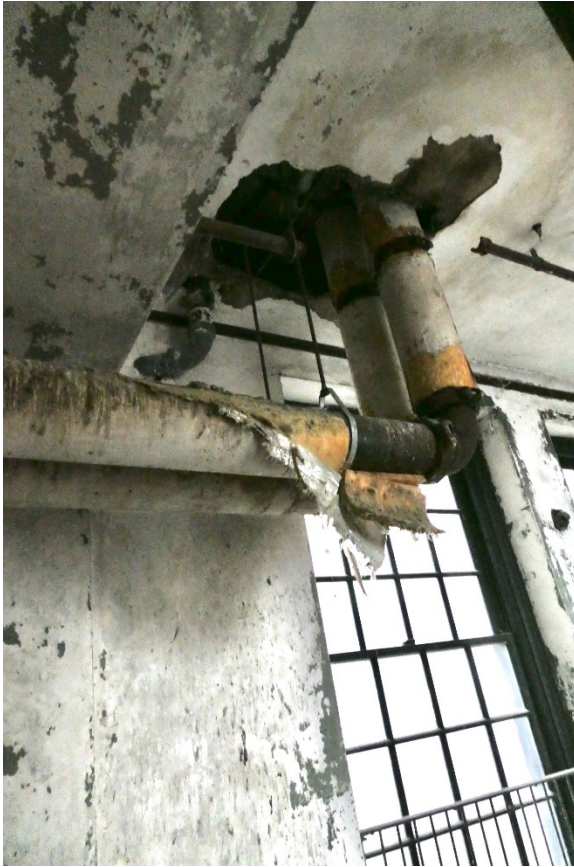
Figure 23. Surfaces losses and disaggregation at plaster surfaces where penetrations were made to accommodate non-historic mechanical equipment on the first level.
