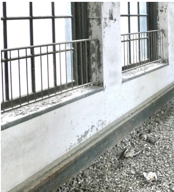
Figure 14. Loss of finishes at metal window guards at the second level of the bridge.
