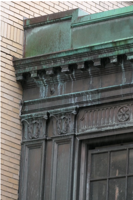
Figure 4. Detail, general atmospheric soil deposition and water staining on copper surfaces.
