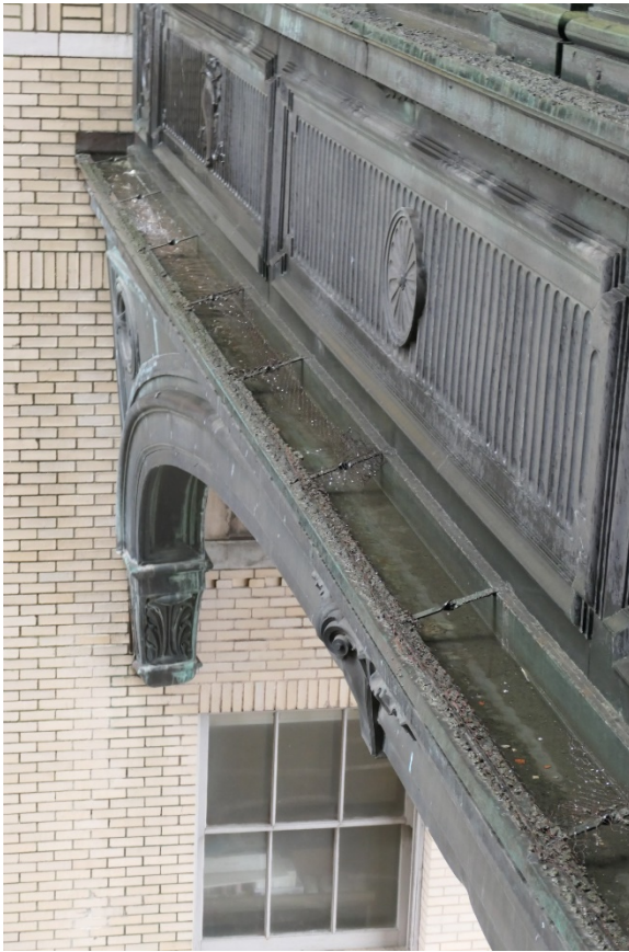
Figure 7. Heavy soil deposition and bird matter at the copper gutter.
