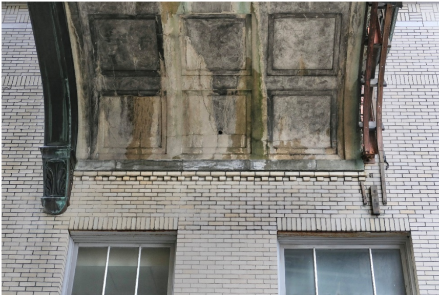
Figure 16. Heavy atmospheric soil deposition, water damage, and biological growth on cement plaster surfaces at the bridge soffit.
