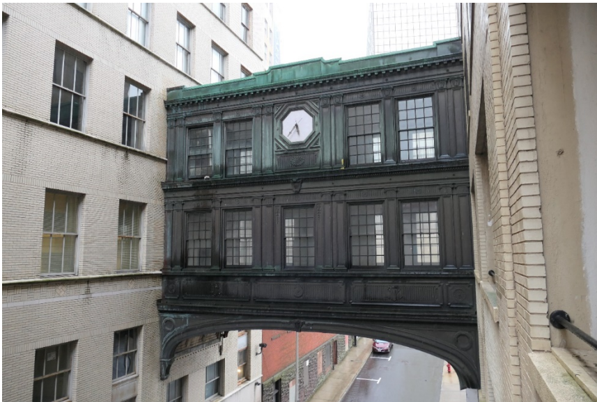
Figure 8. Verdigris patina on copper surfaces is concentrated at the parapet level on the west elevation.
