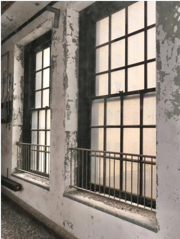
Figure 13. General atmospheric soil deposition, surface losses, and loss of finishes are typical at the kalamein windows. Extensive amounts of pigeon guano are extant on all surfaces especially on the floor at the second level of the bridge.
