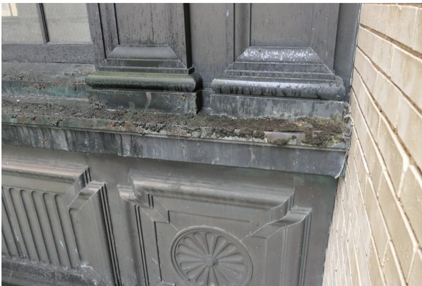
Figure 6. Bird matter on upward-facing surfaces.
