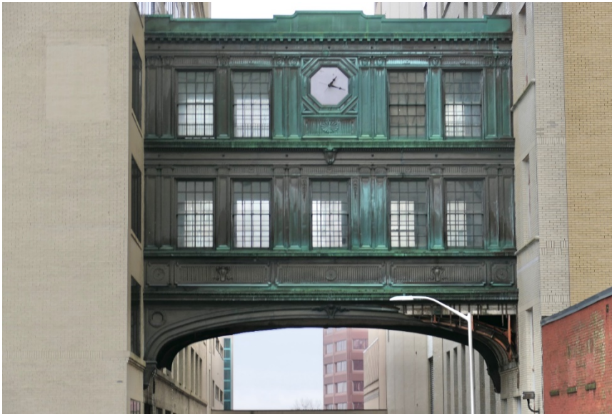
Figure 9. Verdigris patina on copper surfaces occurs throughout each level of the bridge on the east elevation.
