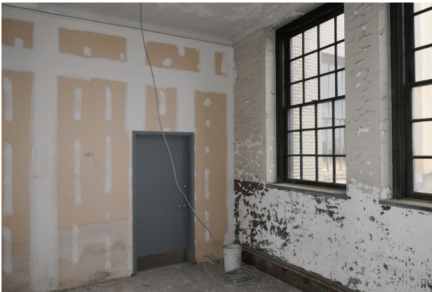
Figure 22. Failing finishes on plaster surfaces on the first level visible at right. Non-historic partition and door at connection to adjacent building visible at left.
