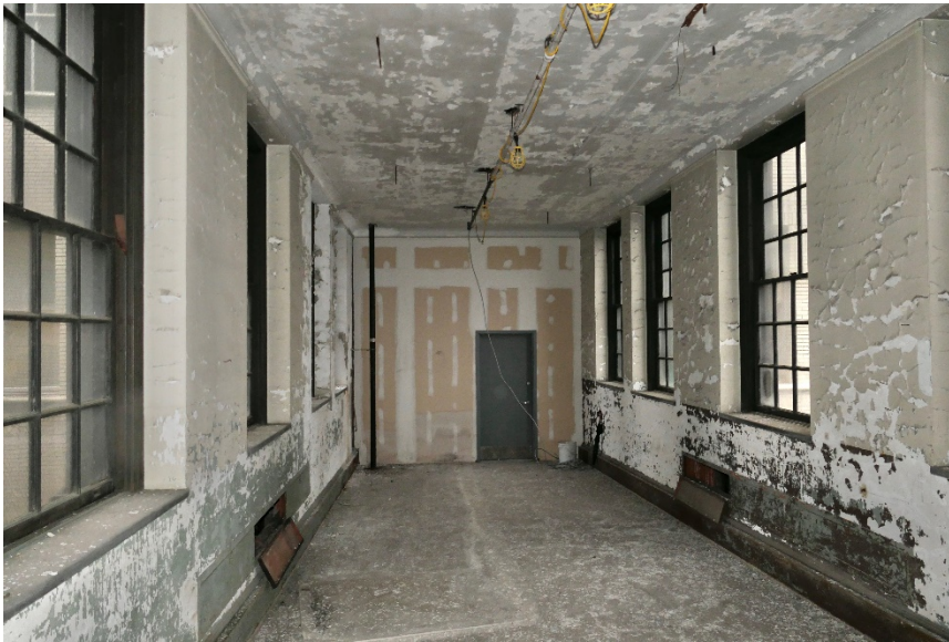
Figure 21. Extensive finish failure at painted plaster walls and ceiling at the first level.
