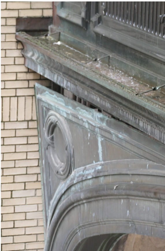
Figure 10. Bent and loose copper cladding is detached from its metal armature at isolated locations.
