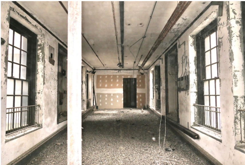
Figure 24. The terrazzo floors at both levels of the bridge are obscured by pigeon guano and debris from failing paint finishes and subsequent construction activity.
