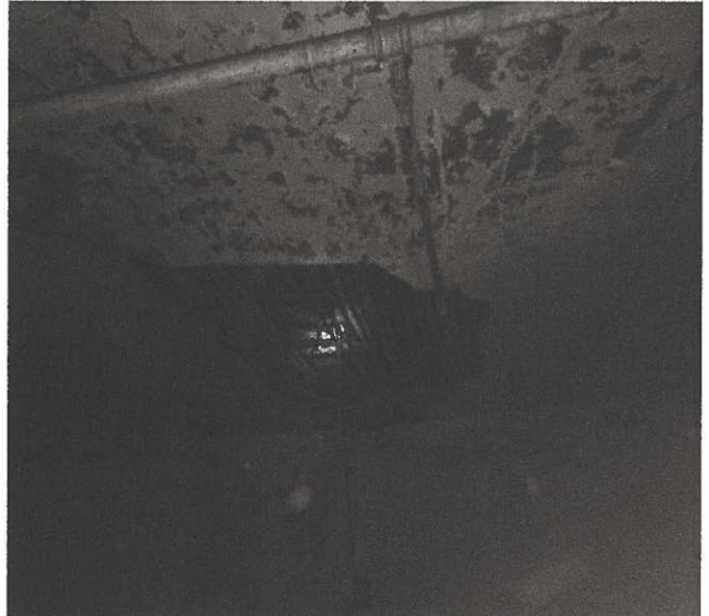
Photo 8 – Large underside spall with exposed steel reinforcement.
