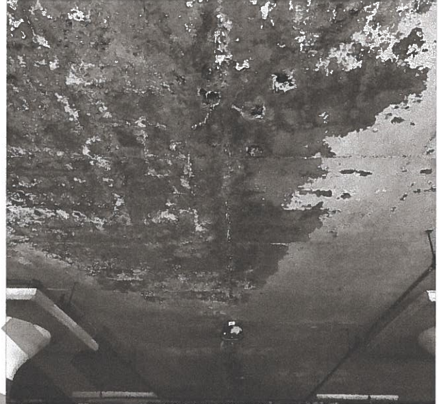
Photo 6 – Deteriorated underside floor slab.
