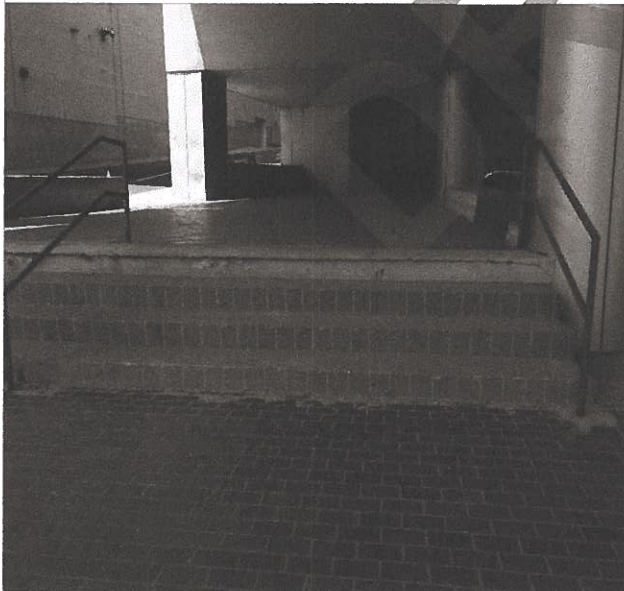
Photo 19 – Minor spalls on Plaza stairs.
