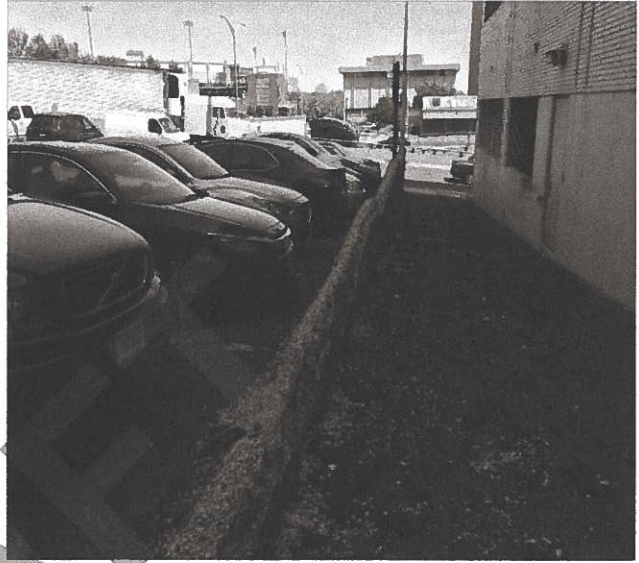
Photo 16 –Morgan Street surface lot walkway weathered asphalt and concrete wall.
