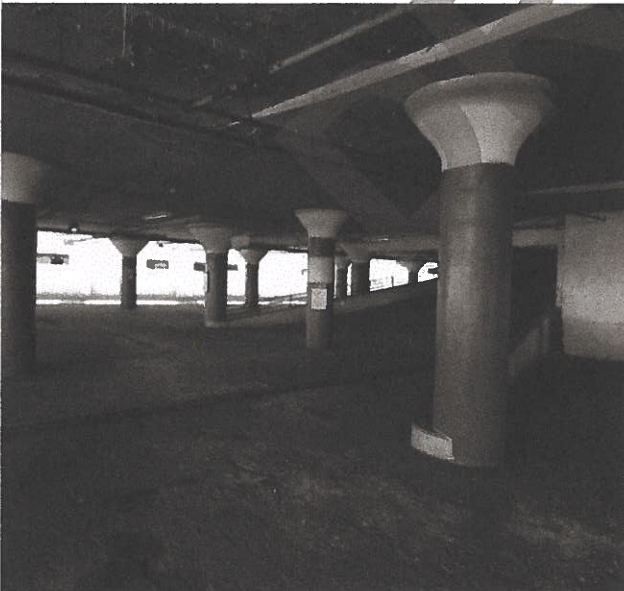
Photo 3 – Topside concrete slab spalls and delamination.
