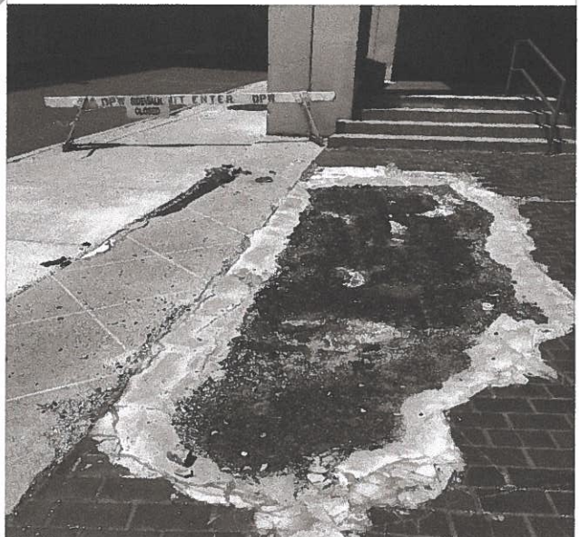
Photo 20 – Plaza surface deterioration.
