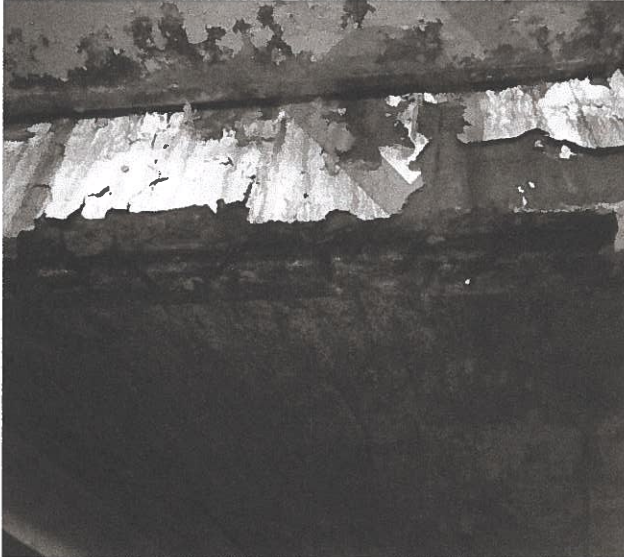
Photo 7 – Random underside beam spall with exposed reinforcing.
