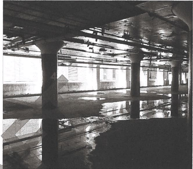
Photo 2 – Ponding on topside slab due to the lack of adequate drainage system.
