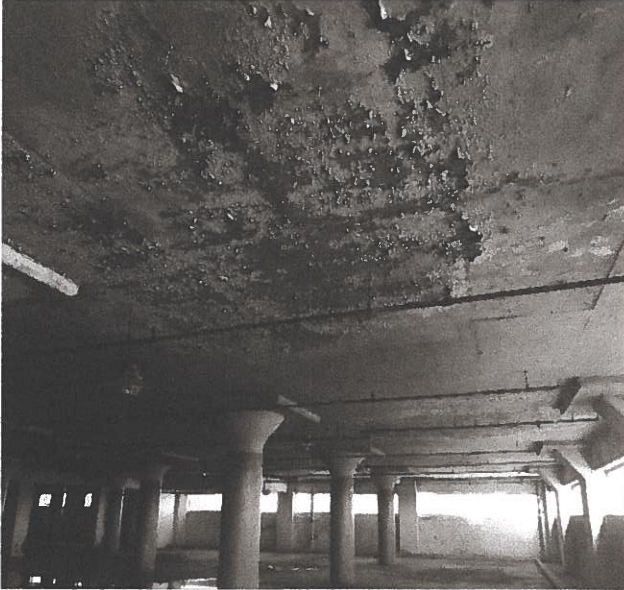
Photo 5 – Typical underside slab delamination.
