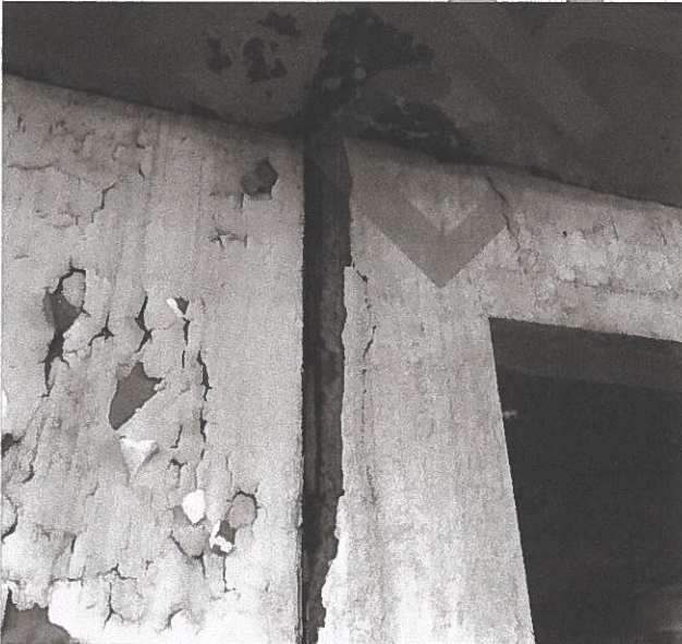
Photo 11 – Column spall with exposed steel reinforcement.
