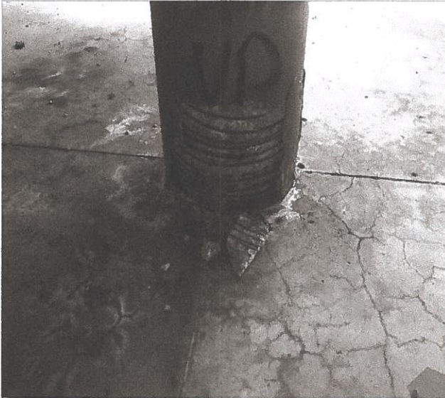
Photo 9 – Spall at column base due to water intrusion. Note the exposed steel reinforcement.
