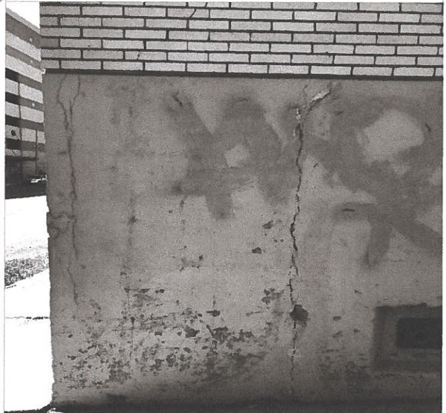
Photo 16 – Cracking and spalling at building base.
