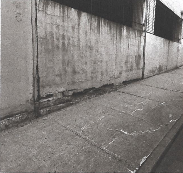
Photo 13 – Water staining and spalling on exterior wall.
