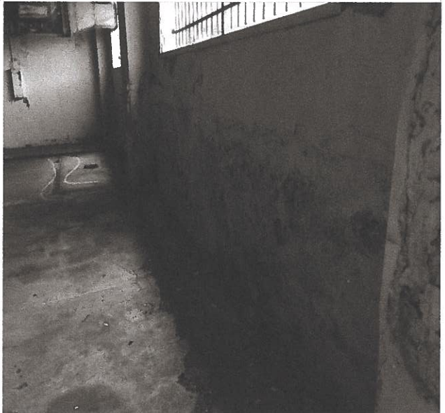
Photo 12 – Column & wall spalling and delamination.
