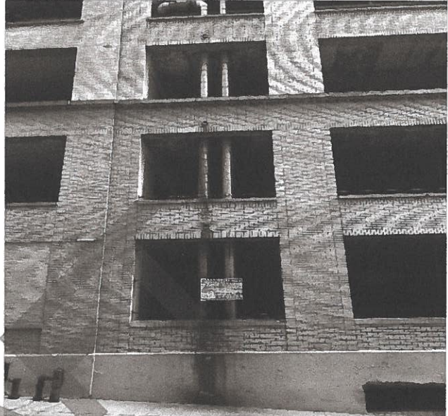
Photo 14 – Staining on exterior brick façade.
