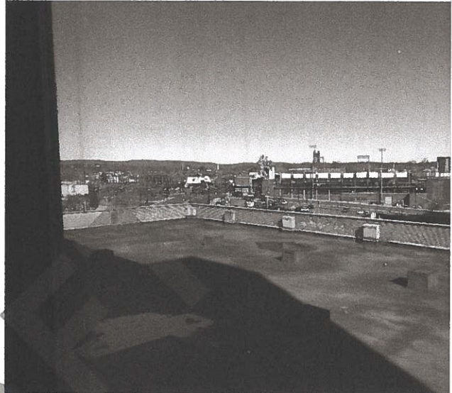
Photo 18 – Minor ponding on garage roofing system. Note the lack of drainage on the Northwest side of roof.
