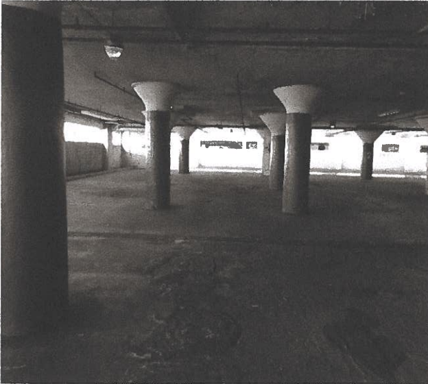
Photo 1 – Delaminated concrete slab. Note the presence of failed bituminous repairs.
