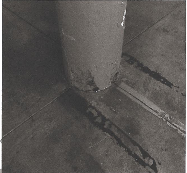
Photo 10 – Column base spalling.
