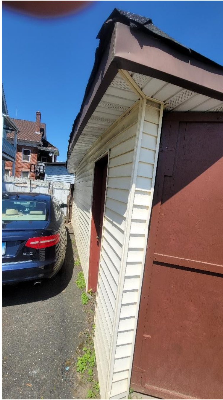
PHOTO #3 LEANING AND BOWED ROOF LINE
