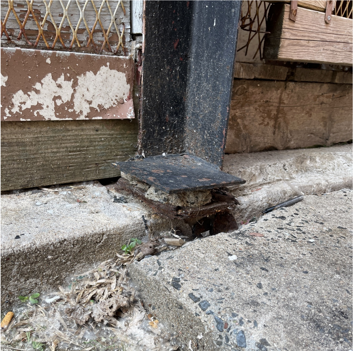
Photo 1: This balcony column base has no anchorage and no apparent foundation.
