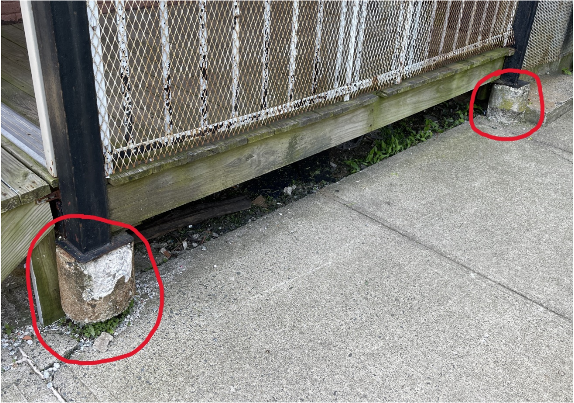
Photo 2: Several columns are lacking anchorage, foundations or have foundation damage.
