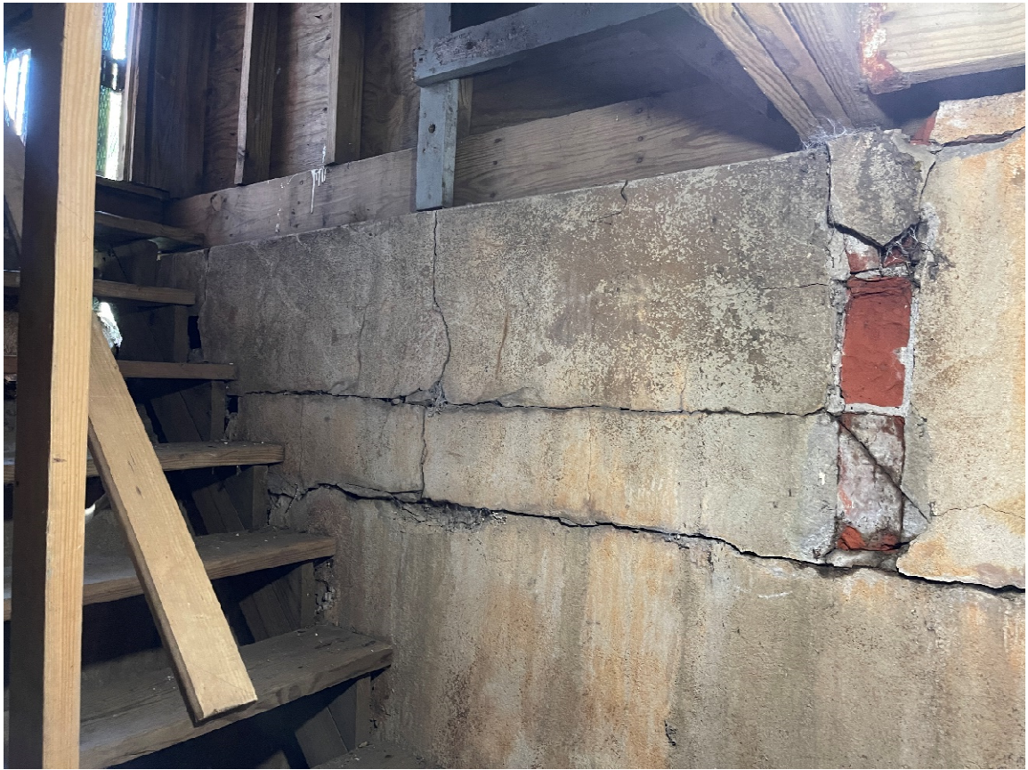
Photo 6: The foundation walls below the balconies are severely cracked and spalled at several locations.
