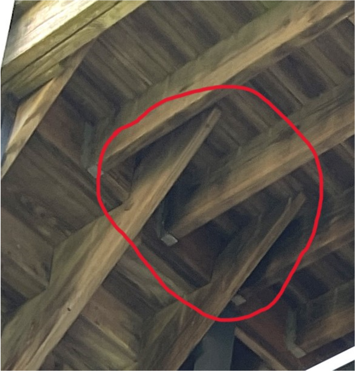
Photo 5: Most of the stair stringers are not adequately connected to the main framing.
