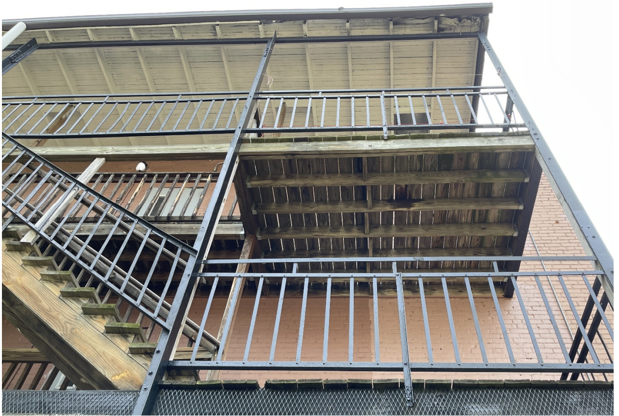
Photo 4: The deck, stairs, railings, and framing are showing signs of deterioration at several locations.
