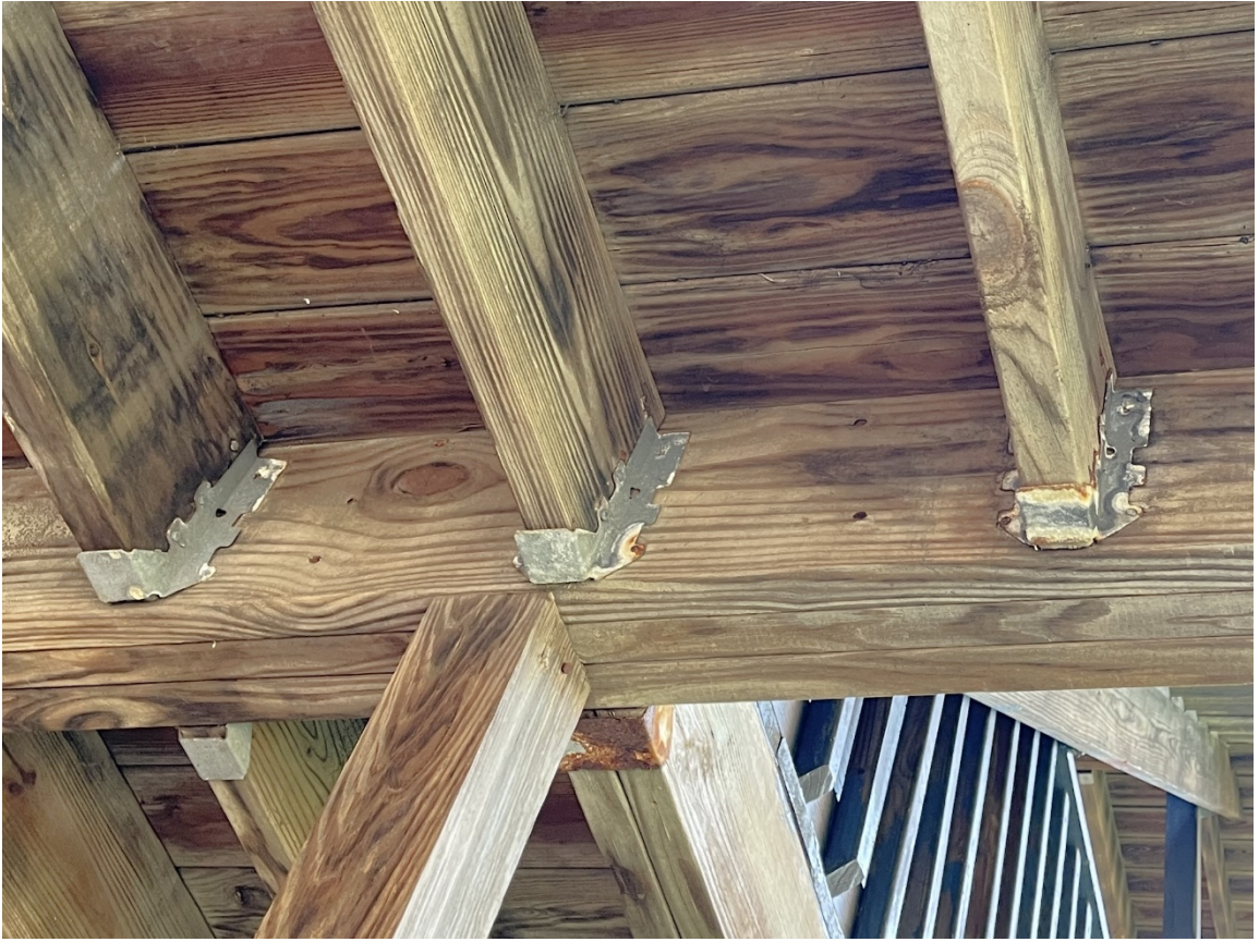
Photo 3: The framing connections are showing signs of deterioration and columns are not sufficiently connected to the girders.
