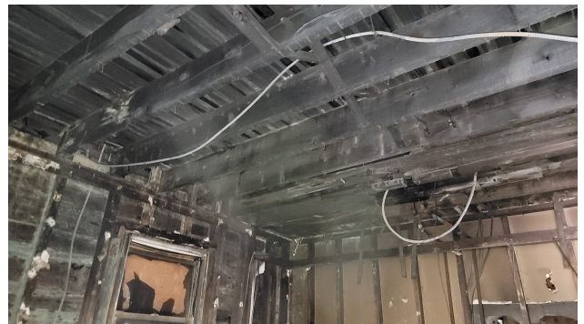
8. 2 nd floor framing smoke staining.
