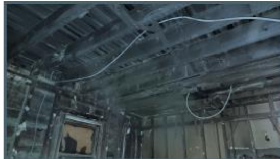
8. 2 nd floor framing smoke staining.
