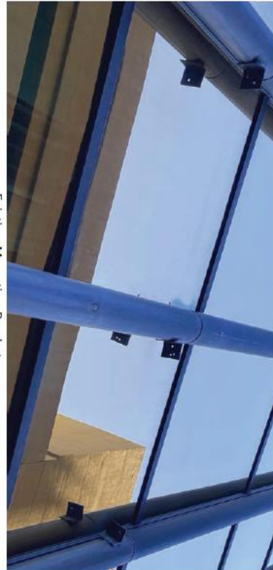
Existing Mounting Brackets
