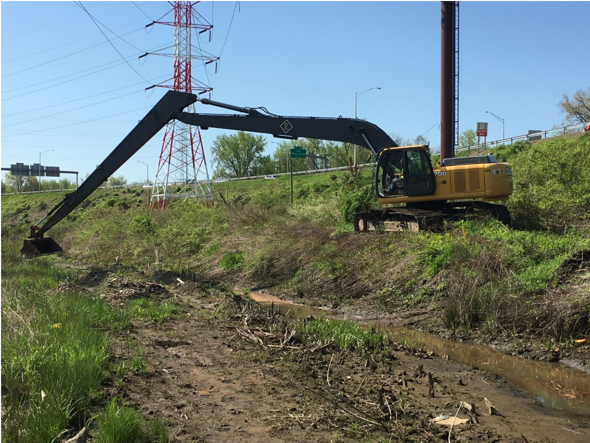
Excavator removing fill material in the northern/central portion of the site looking southwest
