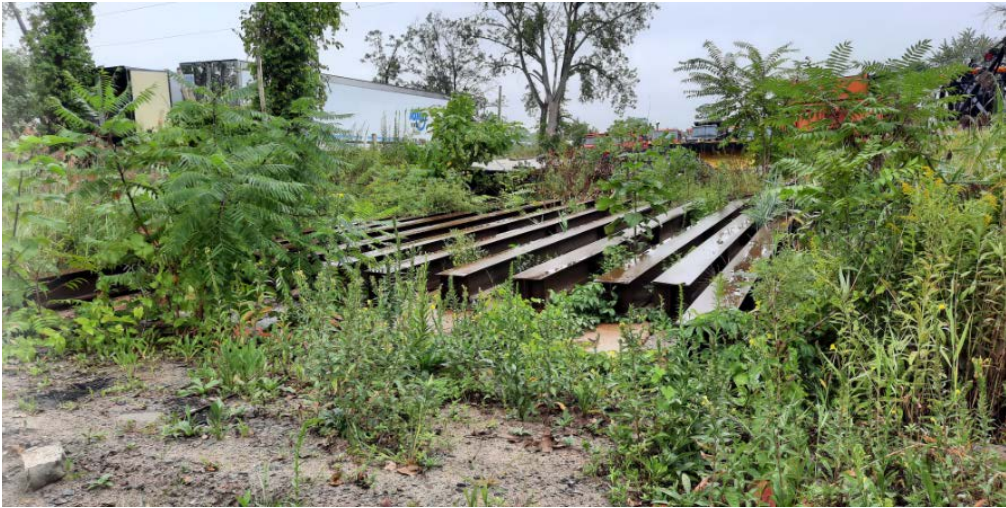
Figure 9. View of bridge components that have apparently been installed across wetlands/watercourse without prior approvals from City Staff, taken 9/10/2020.
